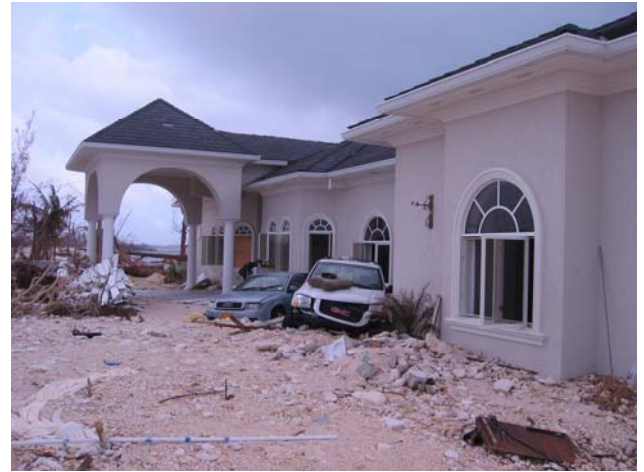
This ICF home in the Cayman Islands withstood the Category 5 devastation of Hurricane Ivan (2004).
