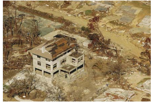
This ICF house was a lone survivor after the storm surge from Hurricane Katrina in 2006.
